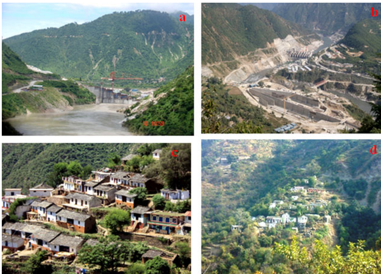
Figure 2. Srinagar Hydroelectric Power Project under construction on the Alakananda River in Garhwal Himalaya (a & b), Villages in the vicinity of Srinagar Hydroelectric Power Project (c & d)
